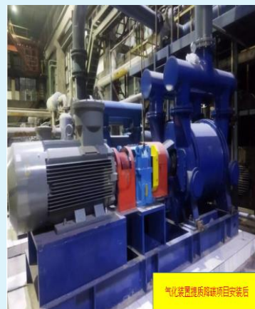
Optimised vacuum pump
