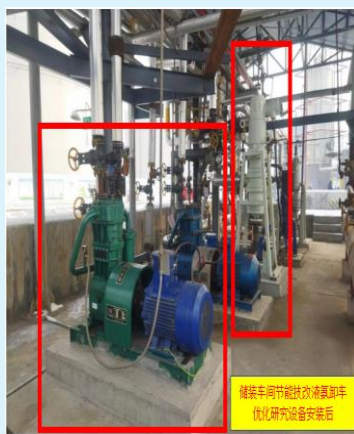
Liquid ammonia unloading pump and unloading ammonia compressor
